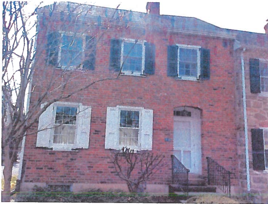
Figure 7. Recently installed Anderson Woodright Series 400 windows at 54 E Wall St –front of house
