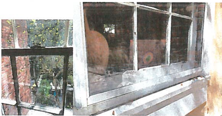
Figure 5. Deteriorating windows at 54 E Wall St = rear of house
