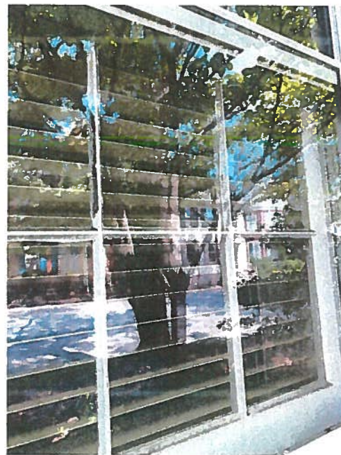
Figure 4. Deteriorating windows at 54 E Wall St = front of house
